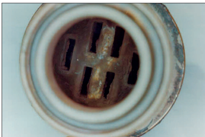
Figure 3: View into the water chamber of a stator bar after some periods of operation. First traces of oxide deposition can be seen in the hollow conductor ends. The water chamber arrangement varies with design.
